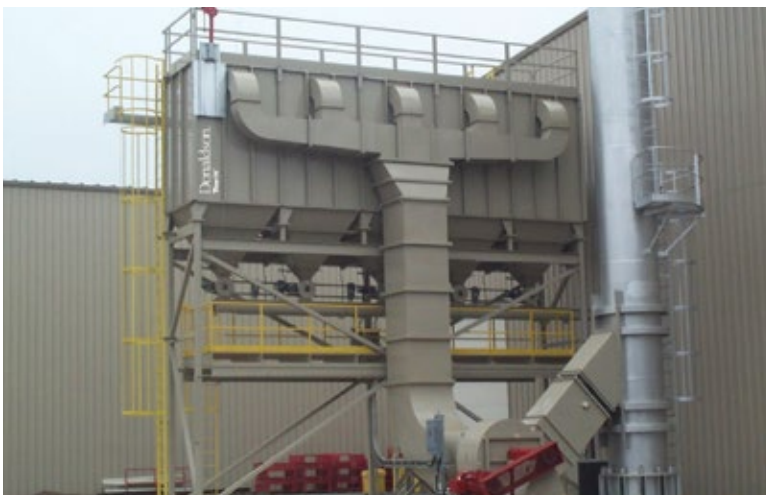
405MBT8 at a Brick Manufacturing Facility
