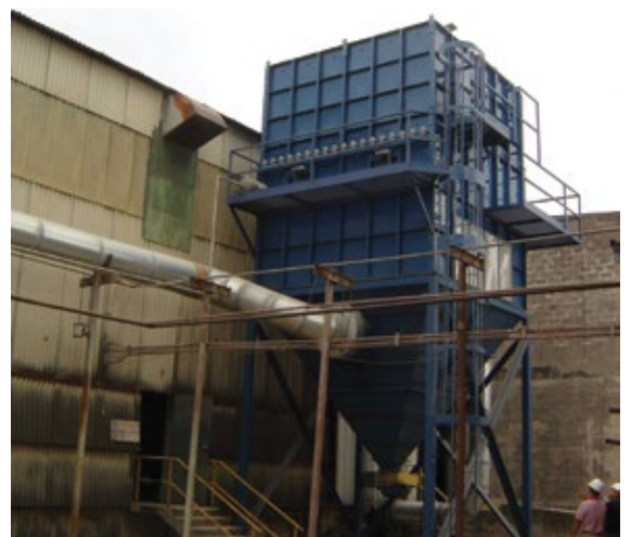
324MBWS10 at a Shingle Manufacturing Facility Collecting Sand
