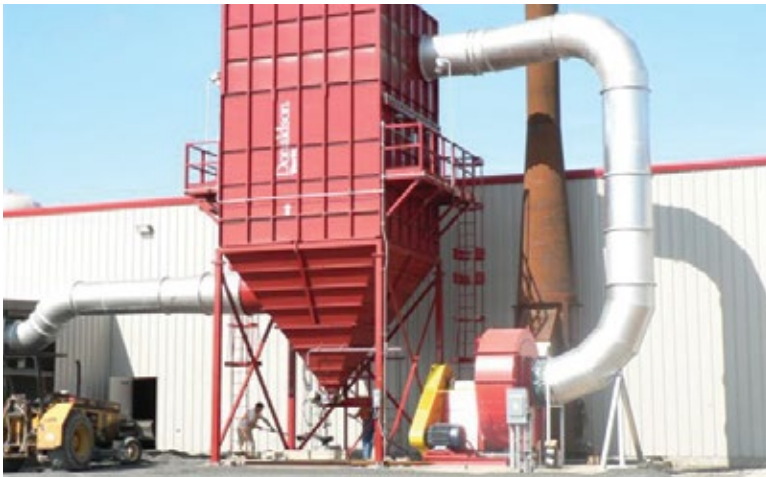
324MBWS10 at a Glass Manufacturing Facility
